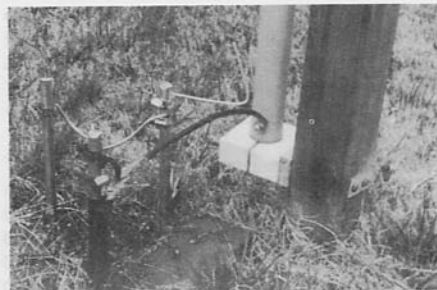
Fig 3—The base of the driven element. The wire projecting from the ground rod and almost touching the base of the antenna element is the horn (air) gap for lightning protection.
